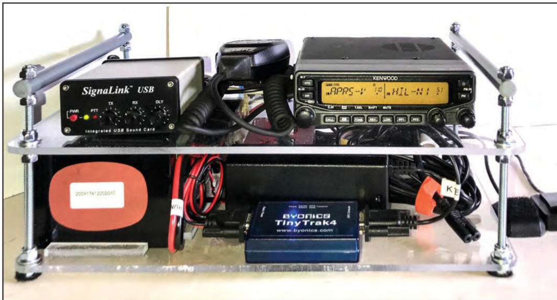
Photo F. Front view of the assembly showing the battery on the left lower level and radio on the right upper level to help balance the weight for carrying. The battery charger is stowed behind the TinyTrak4 TNC.
