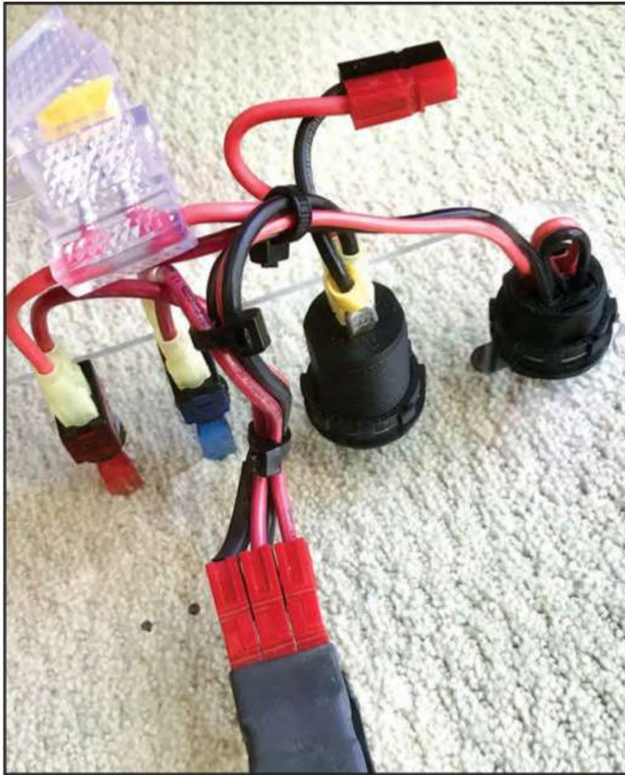
Photo D. Wiring on the underside of the upper level.
