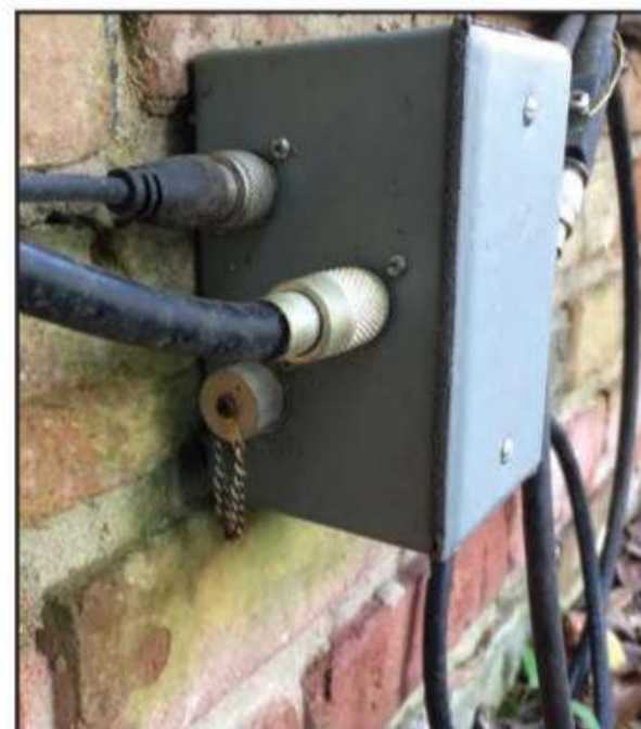
Photo D. Even after a few years of service, the remote switching unit is still ready to connect to a test antenna, allowing a quick comparison of different antennas' performance.
